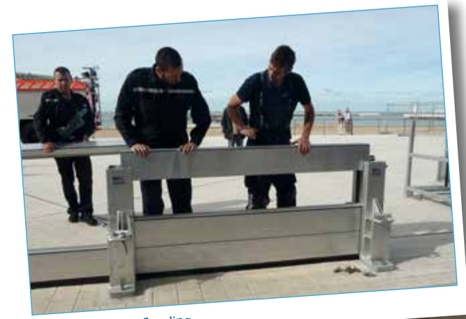
Protection against flooding
